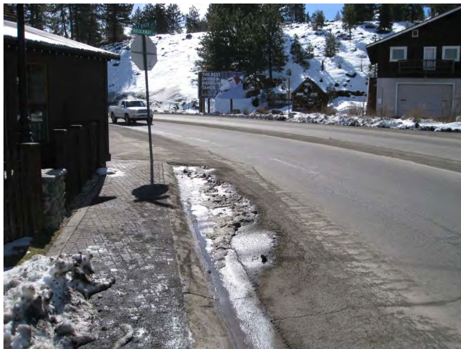
Figure 5-47 Sediment Accumulations on Brockway Road Draining to DSC-TT3
