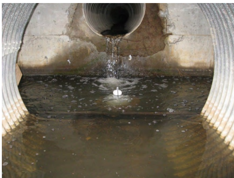
Figure 5-36 Airport Business Park Groundwater Intrusion on November 5, 2012
